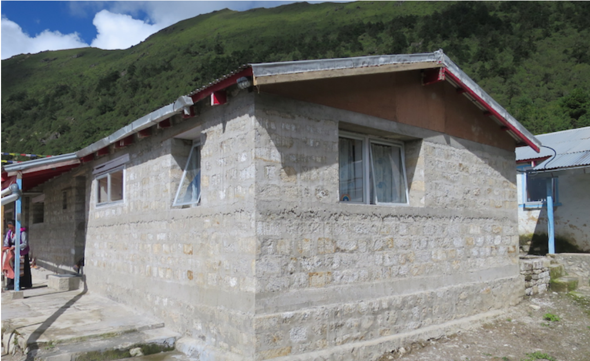
Figure 1: Completion of reconstruction of outer stone masonry wall of the main block (no.2)
