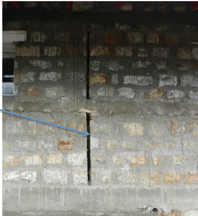
Figure 4: An expansion gap of 2" has been made in the wall at a gap of 12 feet excluding in areas where there are doors. The expansion gap will help in releasing pressure during movements of the building.
