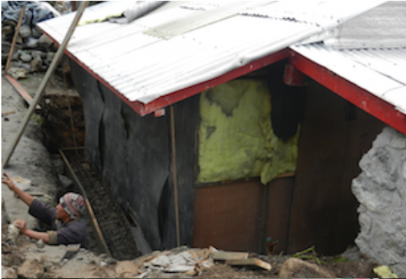
Figure 5: The drug store/X-ray/ultrasound room at the back of the building has been extended and reconstructed
