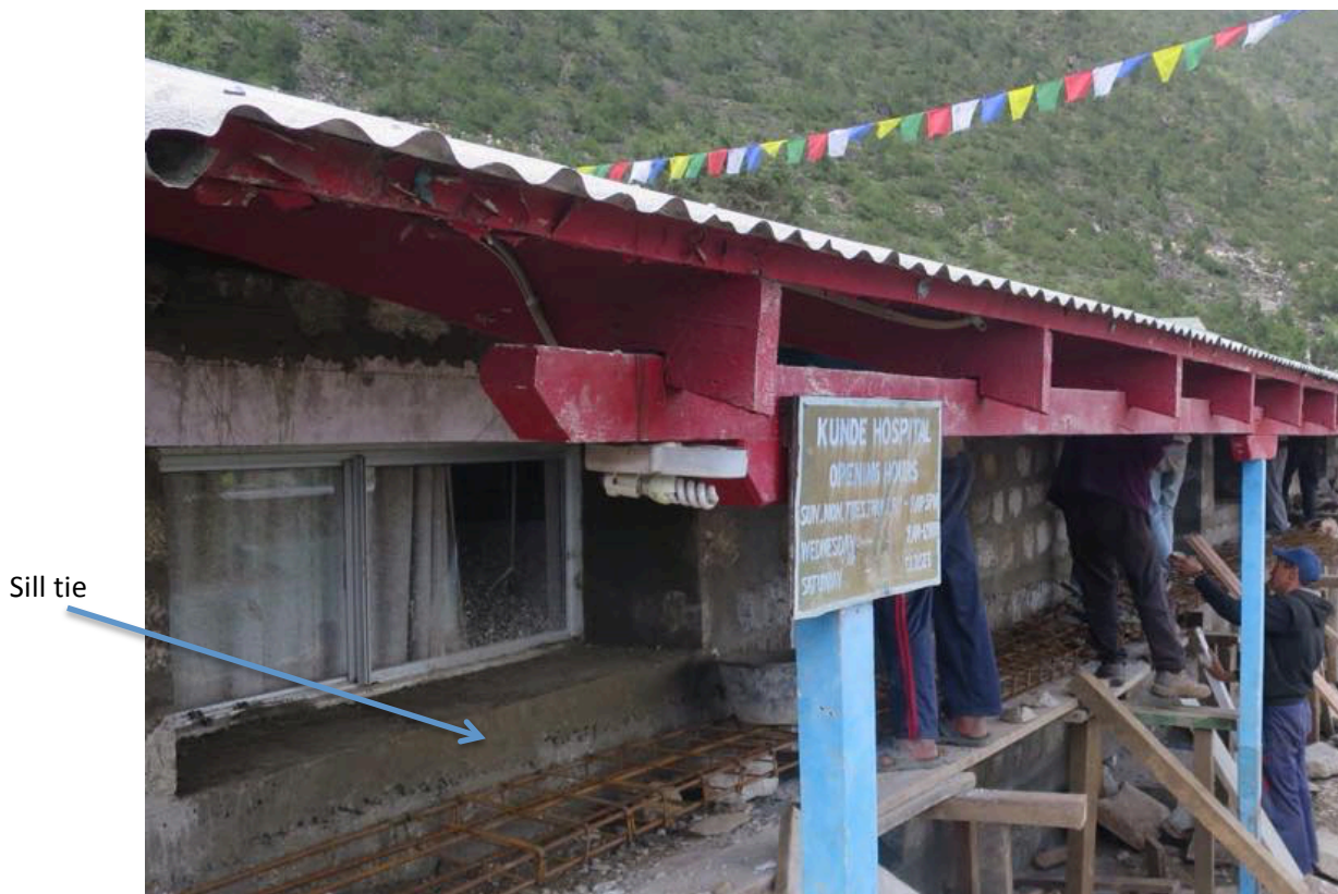
Figure 2: A sill tie made out of iron rod and cement mortar has been placed below the window level to bind the construction materials together to make it earthquake resistant
