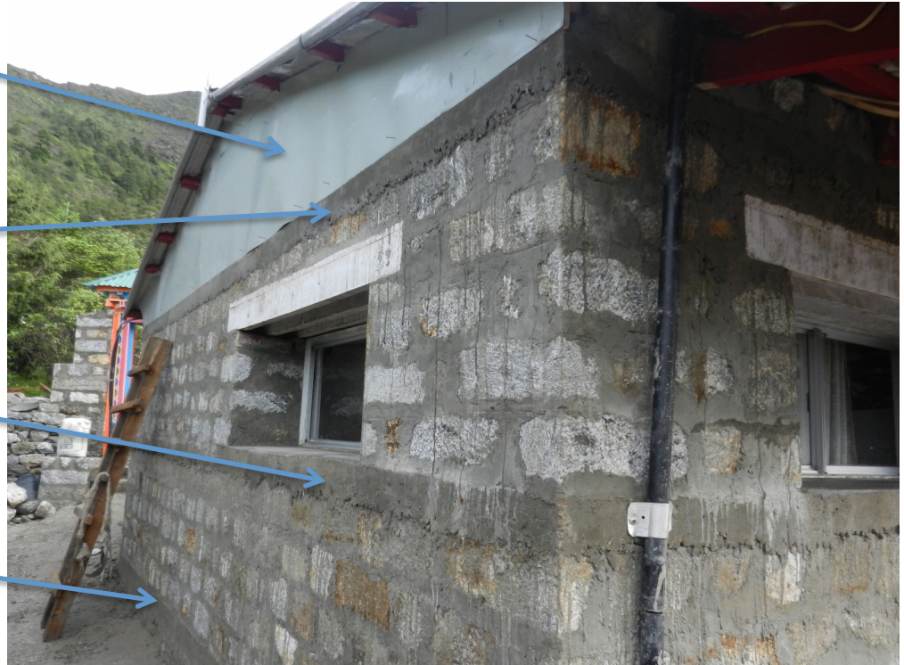
Figure 3: A three-layer tie beam (DPC, Sill and Lentil) has been incorporated in the newly reconstructed stone masonry wall to make it earthquake resistant. Further, vertical rods of 16 mm diameter have been placed at a distance of 8 feet throughout the building.
