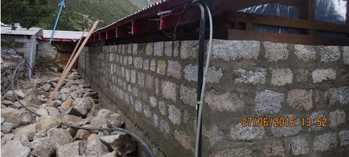
Figure 6: Back view of the reconstruction of stone masonry wall of the main building along with the attached drug store/X-ray/ultrasound room
