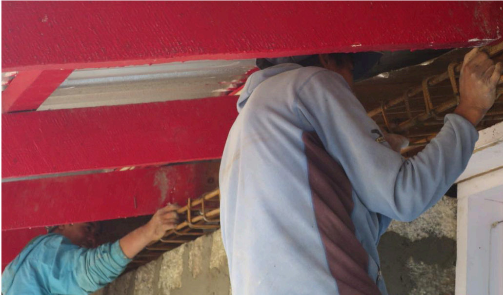
Figure 3: A lentil tie made out of iron rod and cement mortar has been placed above doors and windows level to make the masonry wall more stable
